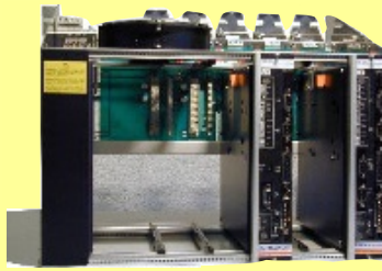
Rack BF-220 & BF-400 and Drives SMTBD1
